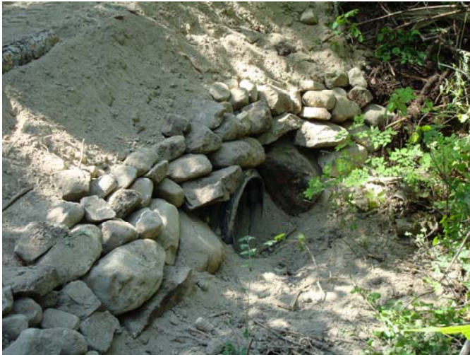
Culverts are installed in wet or seasonally wet draws.
